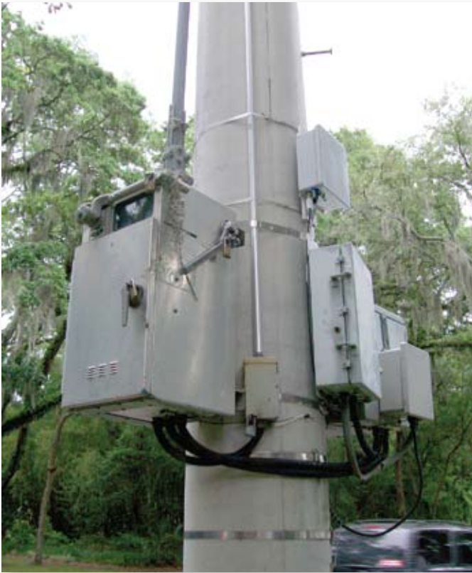
In this complete installation, the DataPAC is attached just above the RTU enclosure with 2½-inch stainless-steel straps.
