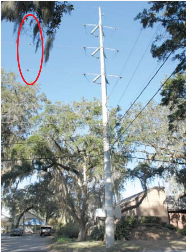
The complete installation with the inconspicuous Linetrackers hanging on the conductors to the left of the switch.
