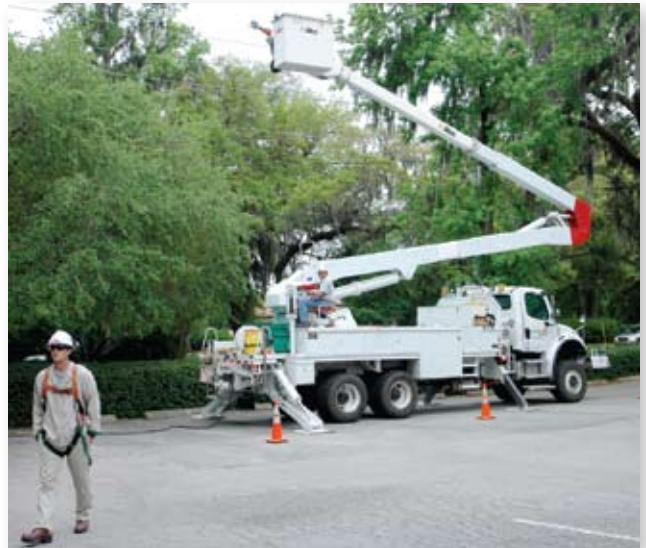
Travis Watts prepares for hot line work on site. He is the crew leader at the local Brunswick Transmission Maintenance Center and performed the Linetracker installation on the conductors.
